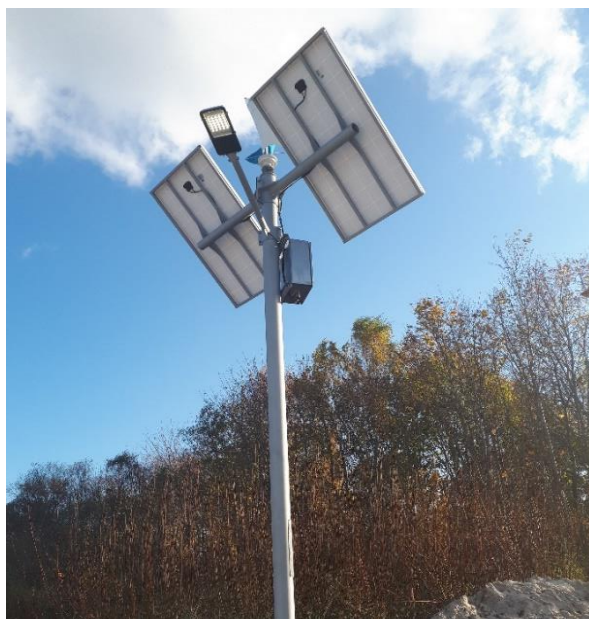
Figure 5. Solar and wind powered autonomous lighting lanterns in Jurmala.
